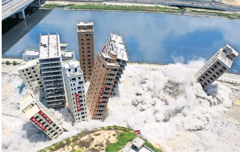
Buildings tumble in a controlled explosion in Shenzhen, where the woes of Evergrande could cause a financial collapse
